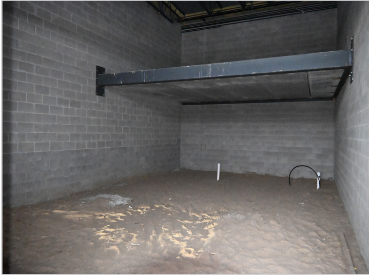
Standard Unit with Dirt Floor and Rough-ins
